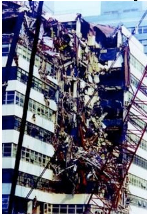
Severe damage done to 30 West Broadway by WTC 7. This building is still under scaffolding in 2006.
